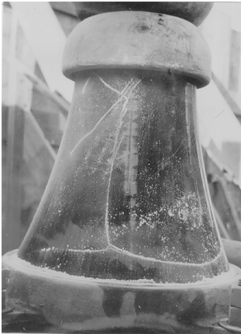
Figure E-24 Results of Statifluxing a Base Insulator. The powder indicates cracks not otherwise visible.
