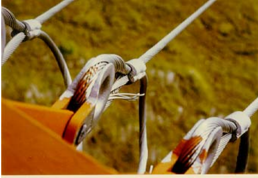
Figure 4-2 Broken strands on TLE.
