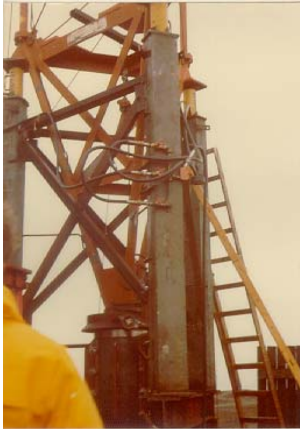
Figure D-8 Hydraulic manifold attached to jacking frame for easy monitoring and security of the lines. Note jacks in place at the top of the jacking frame. A steel collar is attached around the base insulator.
