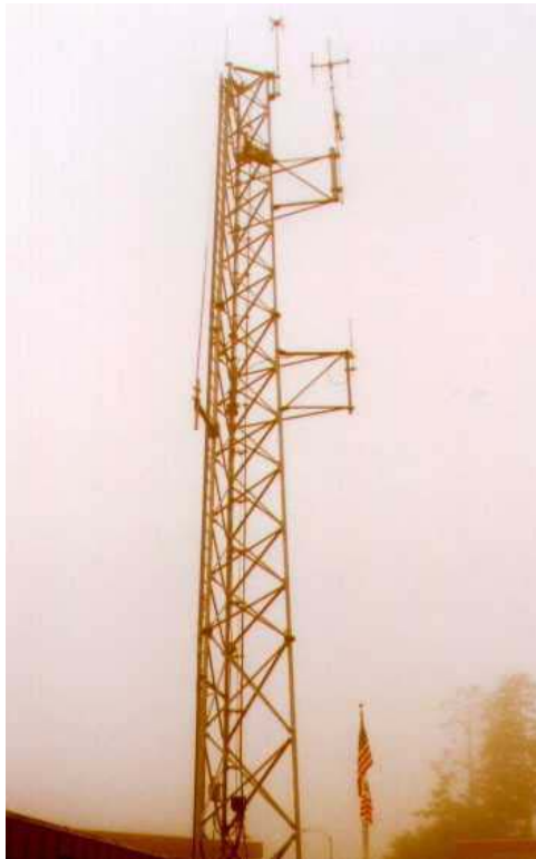
Figure 1-4 60ft Self supporting communications tower.
