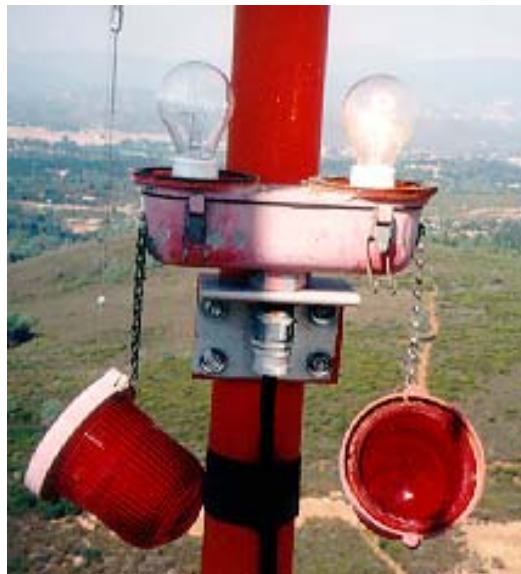
Figure 9-2 Fixed obstruction lights with covers removed for inspection.
