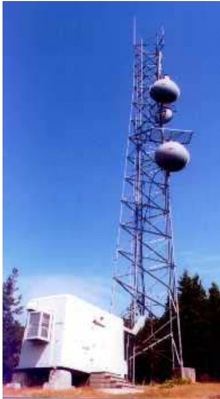
Figure 1-3 Self supporting microwave tower.
