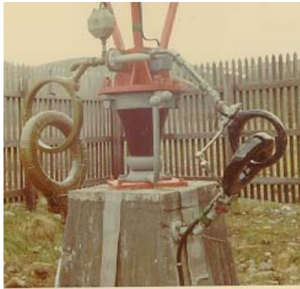
Figure 9-3 Isolation transformers on an energized tower.
