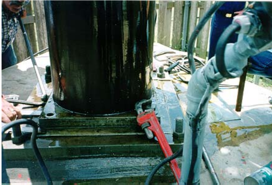
Figure D-10 Removing the bolts that hold down the base insulator. It should be noted that once the tower's weight is removed from the insulator, oil may begin to leak out from under the ceramic portion of the insulator.
