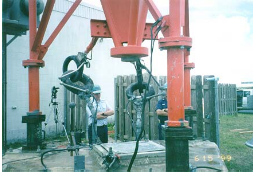
Figure D-5 Jacks, shims, jacking legs, and jacking frame supporting tower after insulator has been removed. Notice shim plates between jack and jacking legs to prevent tower from falling if the jacks fail. Also note that the ball gaps and lighting transformers have been left on the tower but have been adjusted a number of times to provide clearance as the tower was raised.
