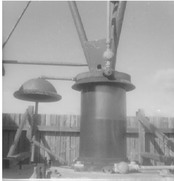
Figure 5-5 Oil filled cylindrical base insulator.
